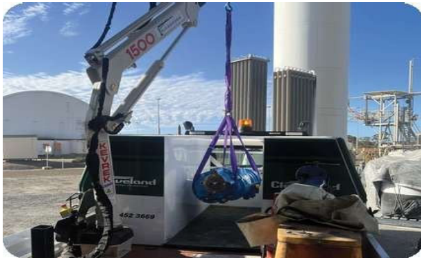
Onsite airend exchange — swapped out remotely, quickly and easily, minimising site downtime.
