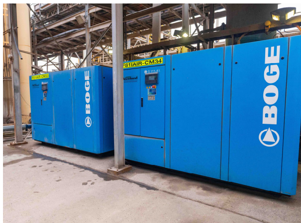
The replacement BOGE S111-4L units installed at KCGM.
