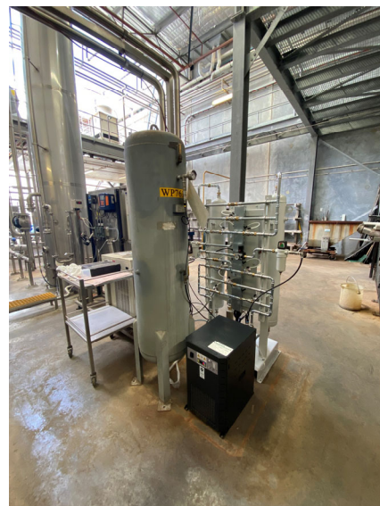
Onsite oxygen generation supporting Asahi's production line.
