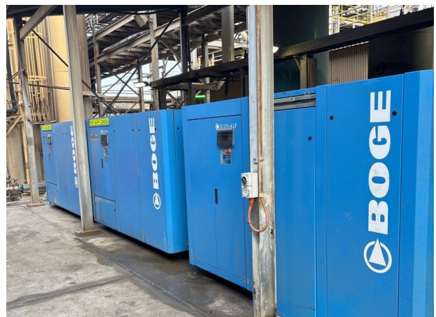
The upgraded compressor row supplying KCGM's flotation plant.
